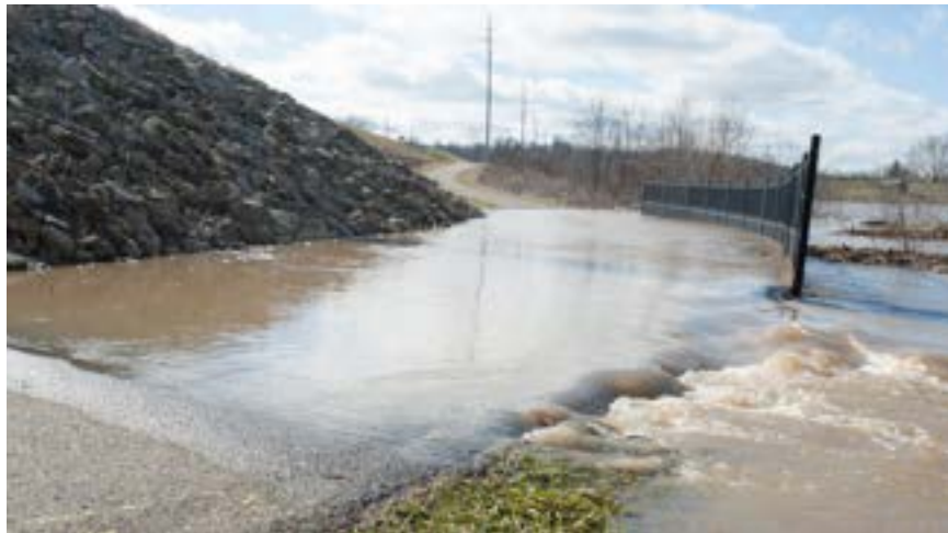
Water damaged roadway in Ross County in 2019. Source: Chillicothe Gazette .
